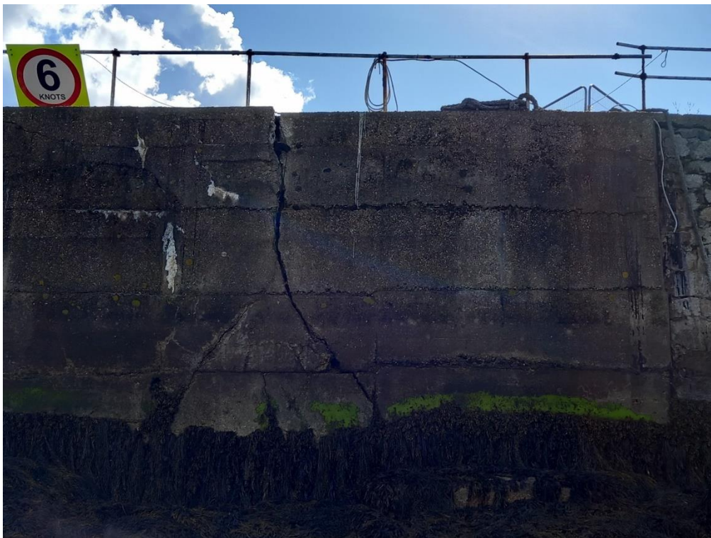
Figure 2-8: Structural failure to the west of the Central Causeway, looking east, Ramboll image 2022
